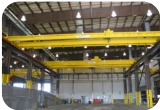
Bridge/ wagon cranes
